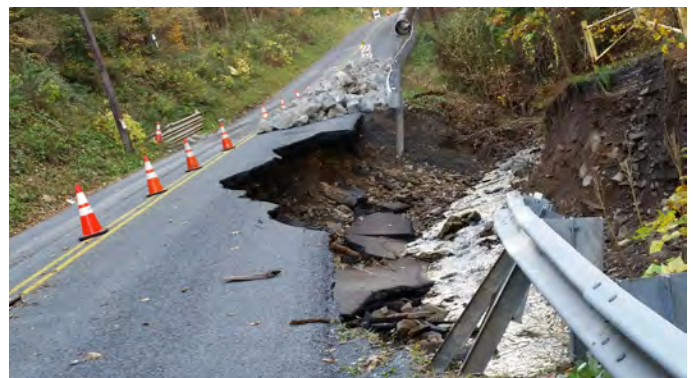
Purdue Mountain Road Collapse in 2016
