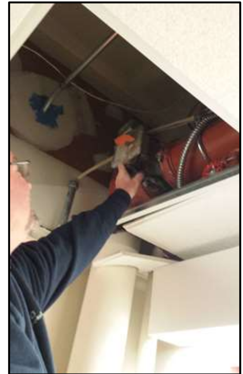
Figure 55. The Schlow Library's fire sprinkler system required an update after pipes froze and burst during a February 2015 cold snap.
